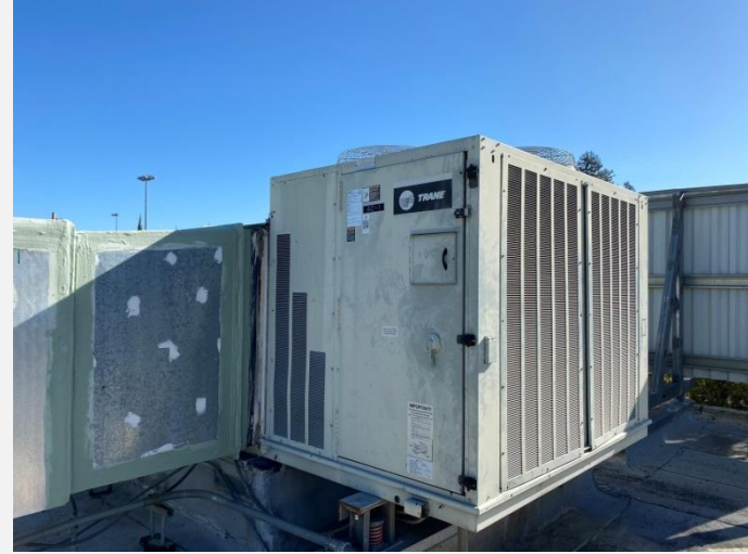
(E) UNITS & DUCTWORK To be demolished
