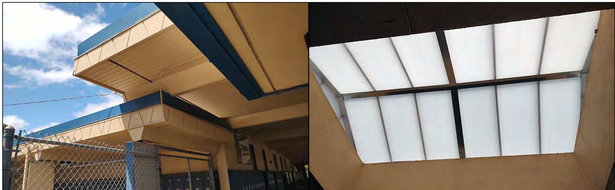
1970-1971 additions. Left : decorative motif on covered walkways; right : skylight at the west side of the quad
