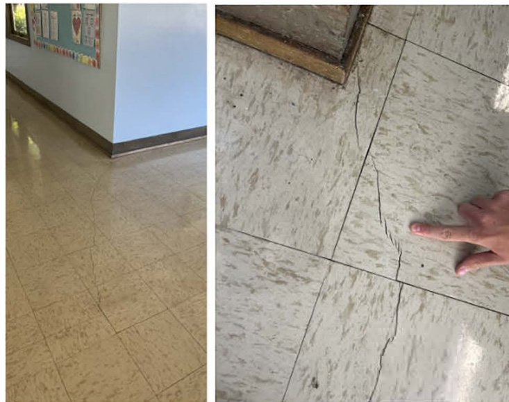
Location 2 - Cracked linoleum floor in main building hallway exhibiting an echelon fractures. Cracks extend across entire hallway along northwest trend.
