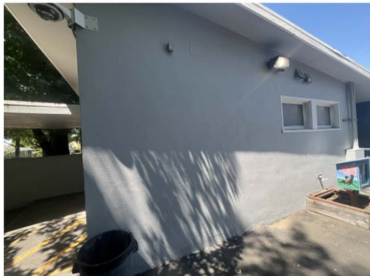
Location 3 - View to north of damaged stucco at south corner of main building at location of deformation zone observed in Trench T-4 and approximately on strike with mapped fault and locations 1 and 2.
