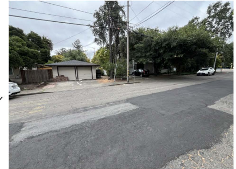
Location 4 - View to south of severely damaged concrete driveways. Most of the concrete flatwork in the surrounding area is older, but in reasonably good condition without similarly prominent or extensive damage.
