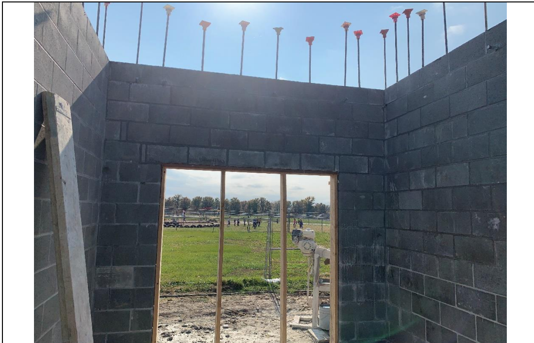
Description Looking at south cmu wall top at corridor no. 203 at Second Grade Wing, where wall is laid 8" too high 3
