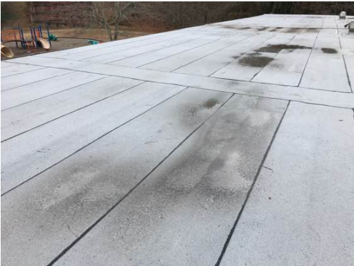
Roof Ponding. Slope To Gutters
