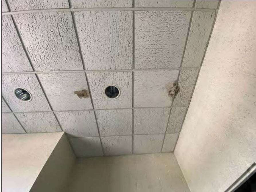
25 - Potential mold and water damage on the first floor
