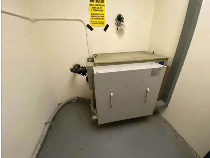
29 - Elevator room with hydraulic fluid reservoir on the second floor
