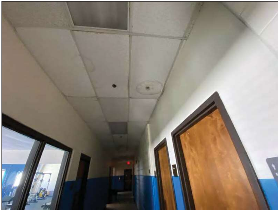
46 - Water damage on the first floor
