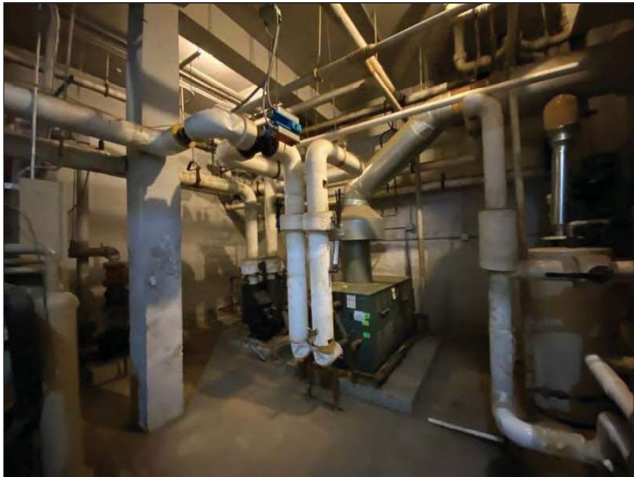
32 - View of mechanical room in the basement area
