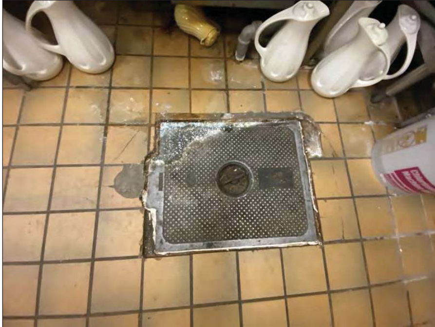
19 - Grease trap in the kitchen
