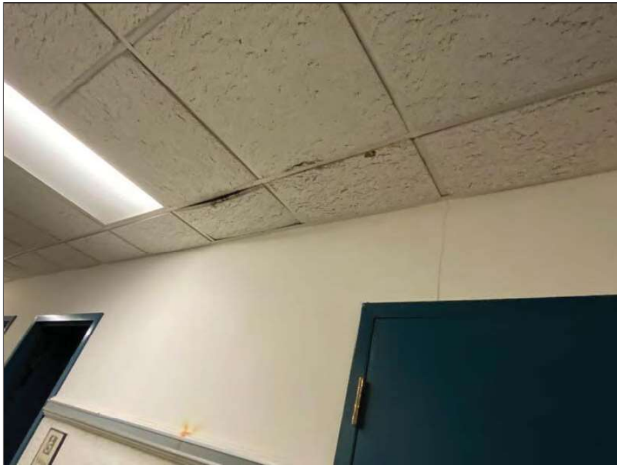
30 - Potential mold and water damage on the second floor
