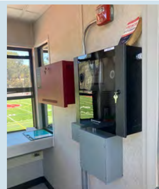
San Rafael High School campuswide alarm
