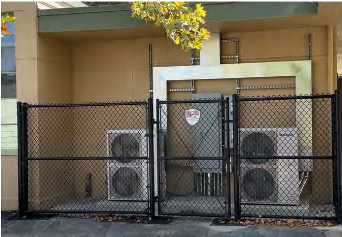
San Pedro HVAC Units
