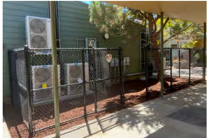
San Pedro HVAC Units
