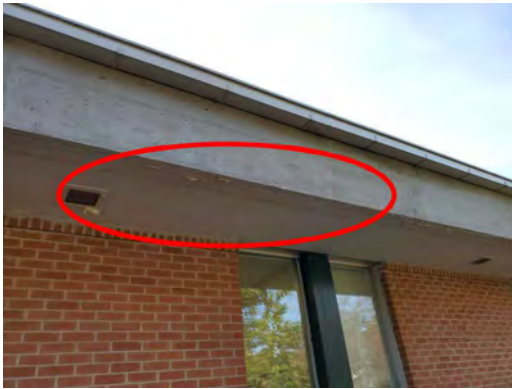
Peeling Paint At Overhang
