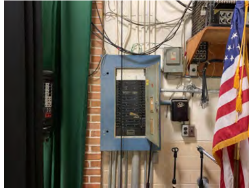
Electrical Panel It States Needs To Be Replaced
