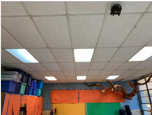
Existing Fluorescent Light Fixtures Should Be Replaced
