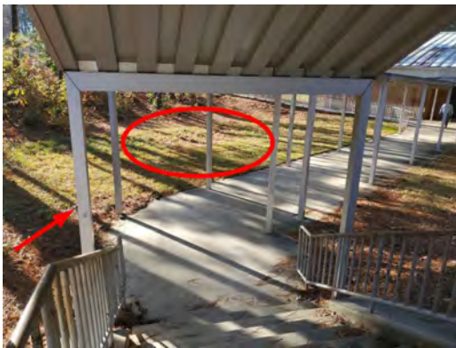
Site Drainage Issue Water Runoff From Stairs With A Steep Slope
