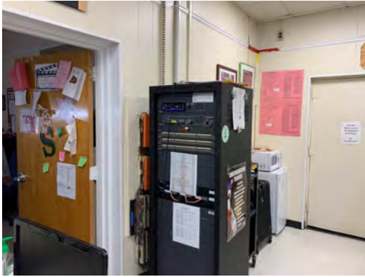
Existing Intercom System To Be Replaced
