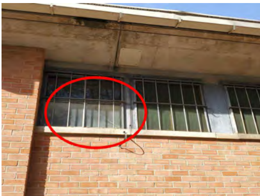
Broken Glass Outside Kitchen
