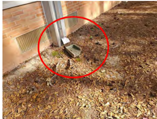
Damaged Metal Downspout And Add Splash Block
