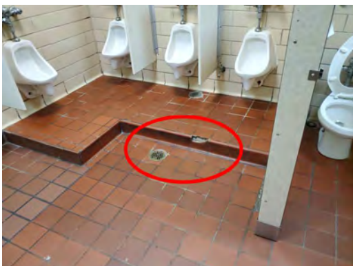
Damaged Tile Floor
