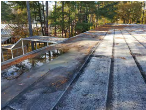
Ponding Water On The Roof
