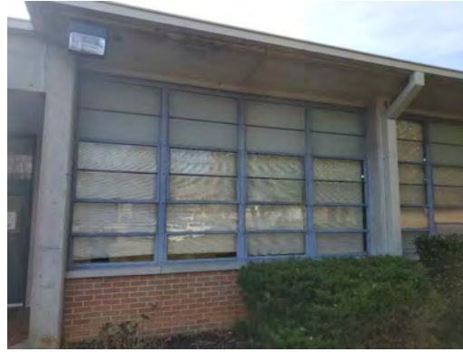
Typical Windows Beyond Useful Life
