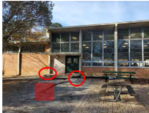
Recommend To Add A Concrete Pavement To Prevent Overflow Of Water From The Metal Downspouts
