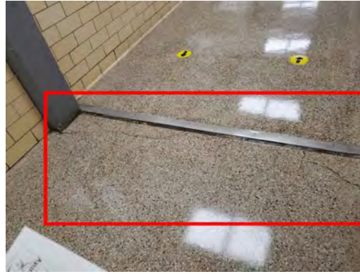
Damaged Terrazzo Floor
