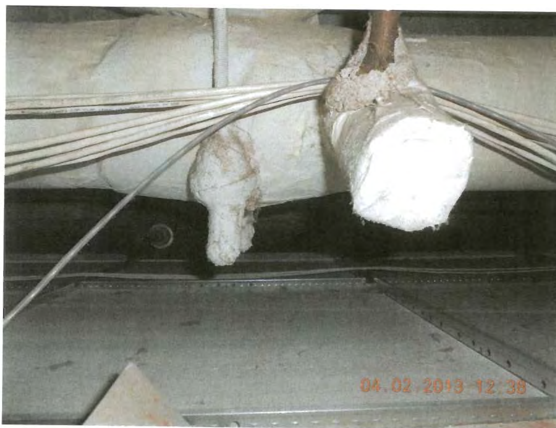
Photo #8 – White putty material on piping
