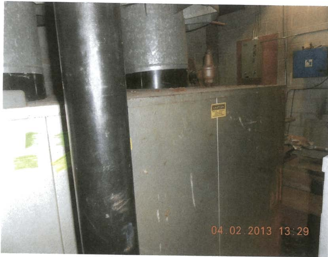
Photo #9 – Boiler – PACM*
