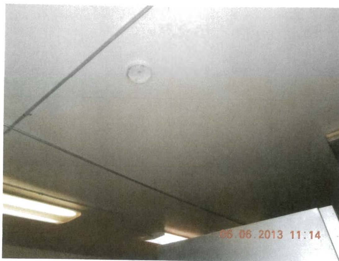
Photo #4 – Plaster - PACM*
