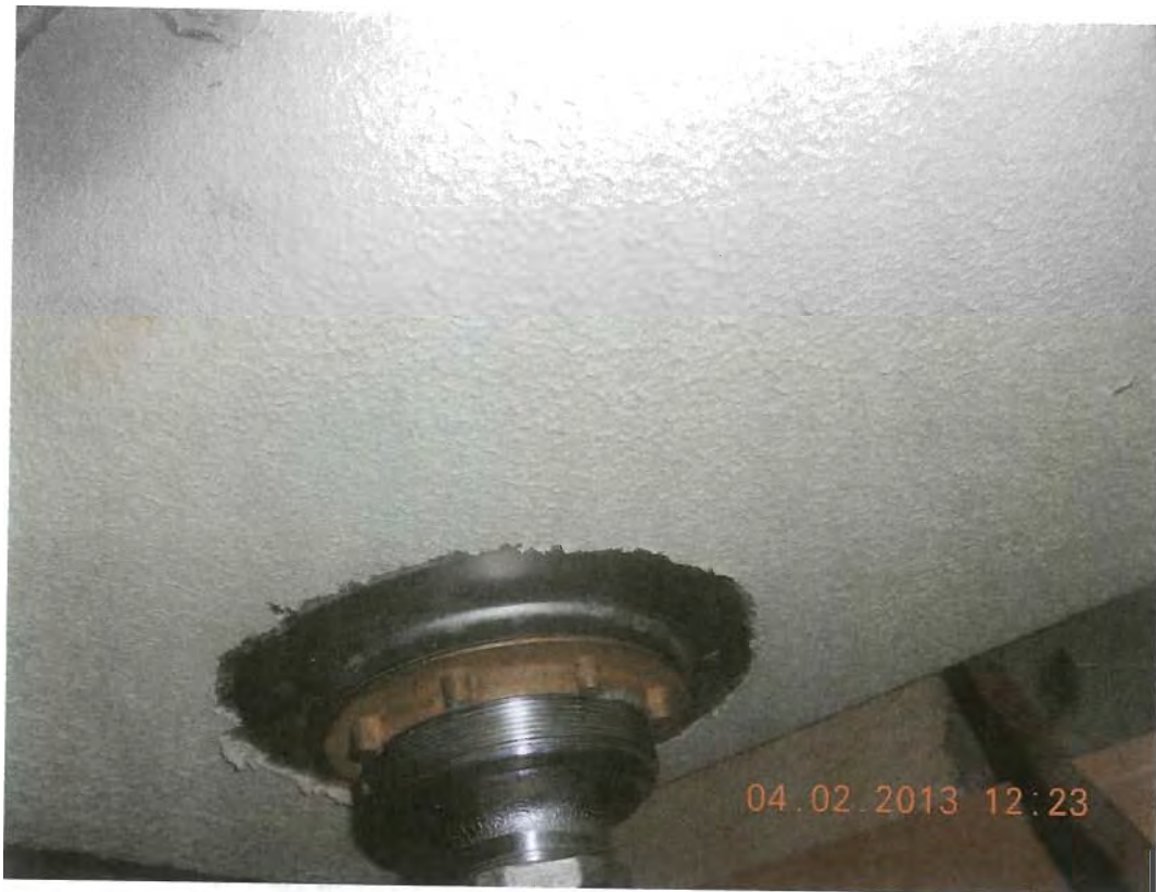
Photo #5 – Sink mastic – white
