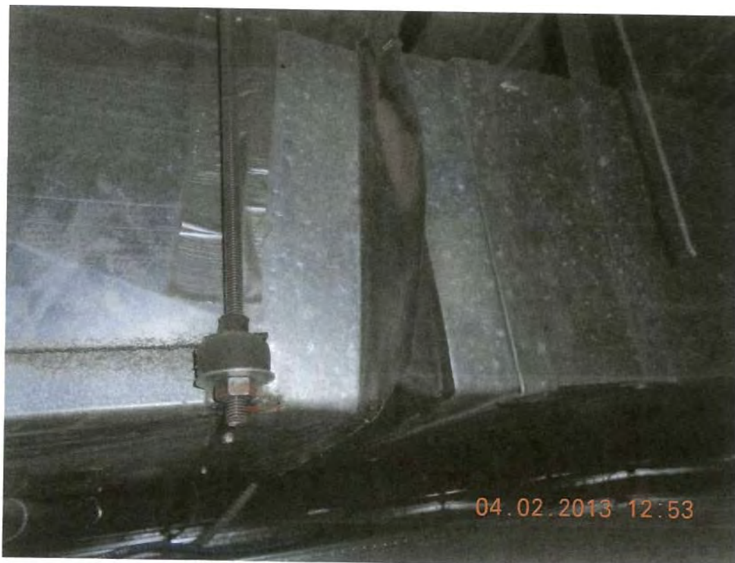
Photo #6 – Vibration Dampeners – PACM*
