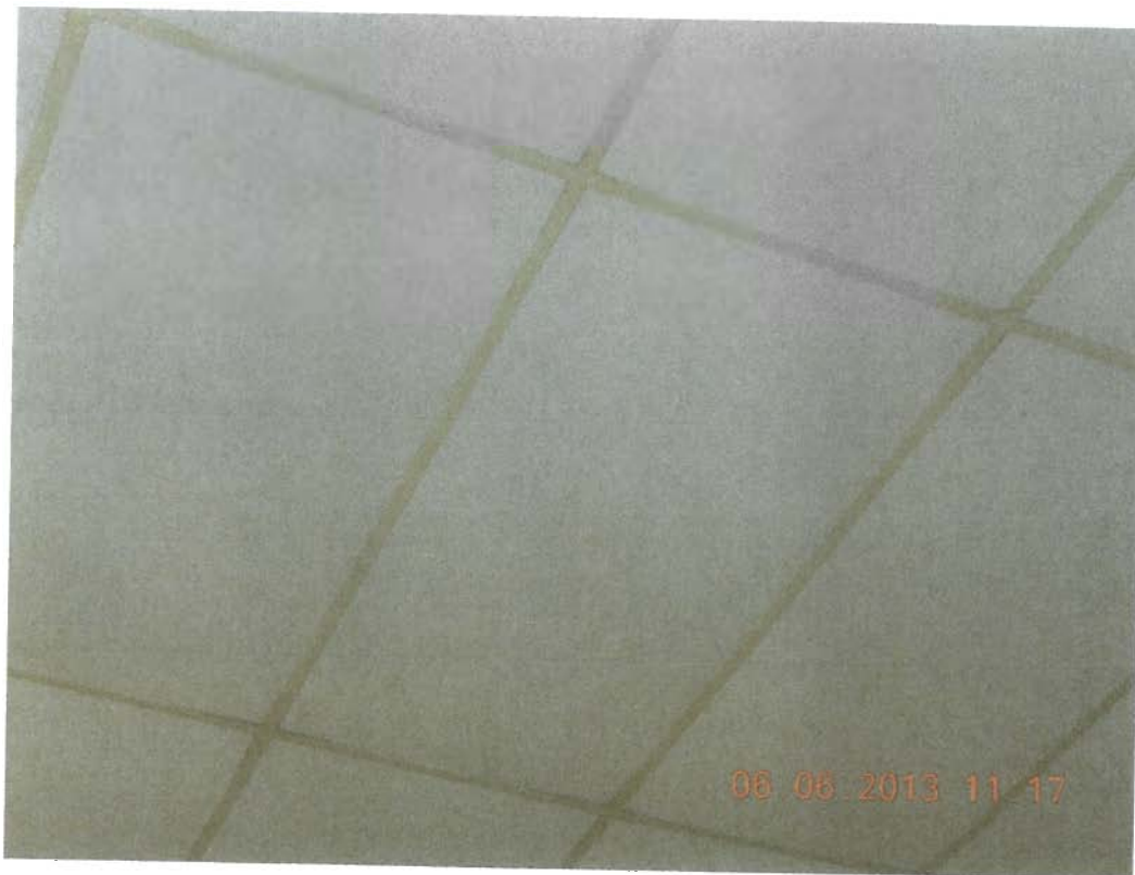
Photo #14 – 2'x 4' drop in ceiling tile – small and large holes
