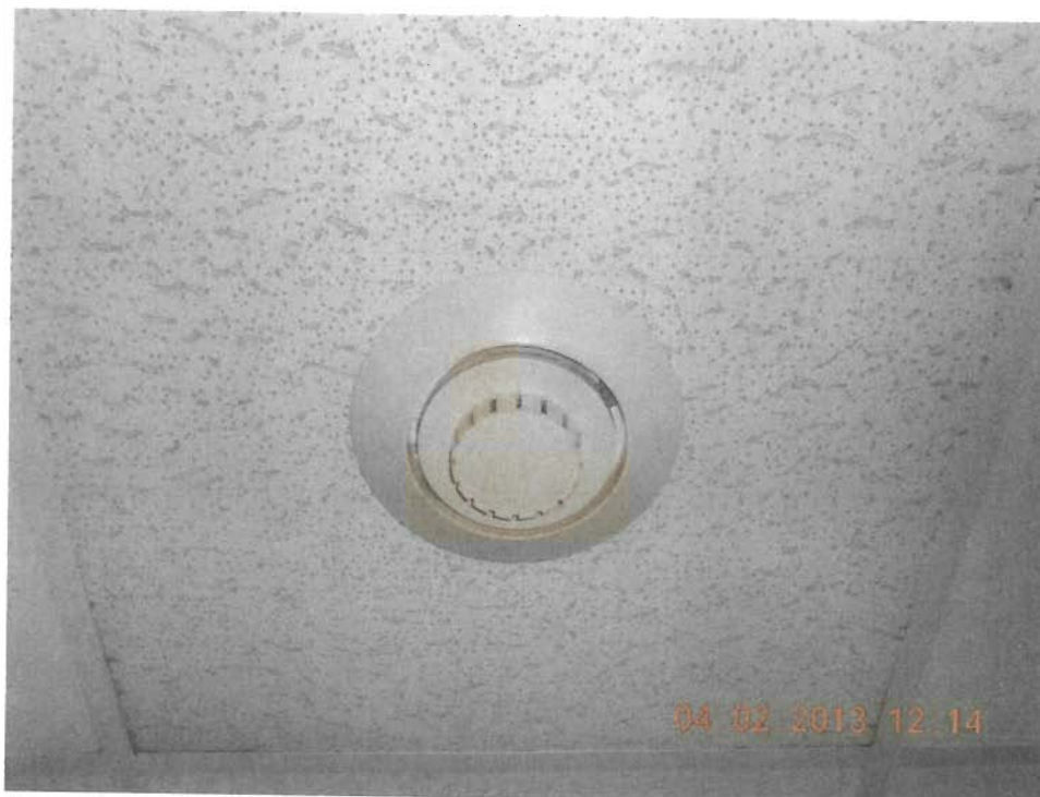
Photo #2 – 2' x 2' drop in ceiling tile – more holes with long fissures
