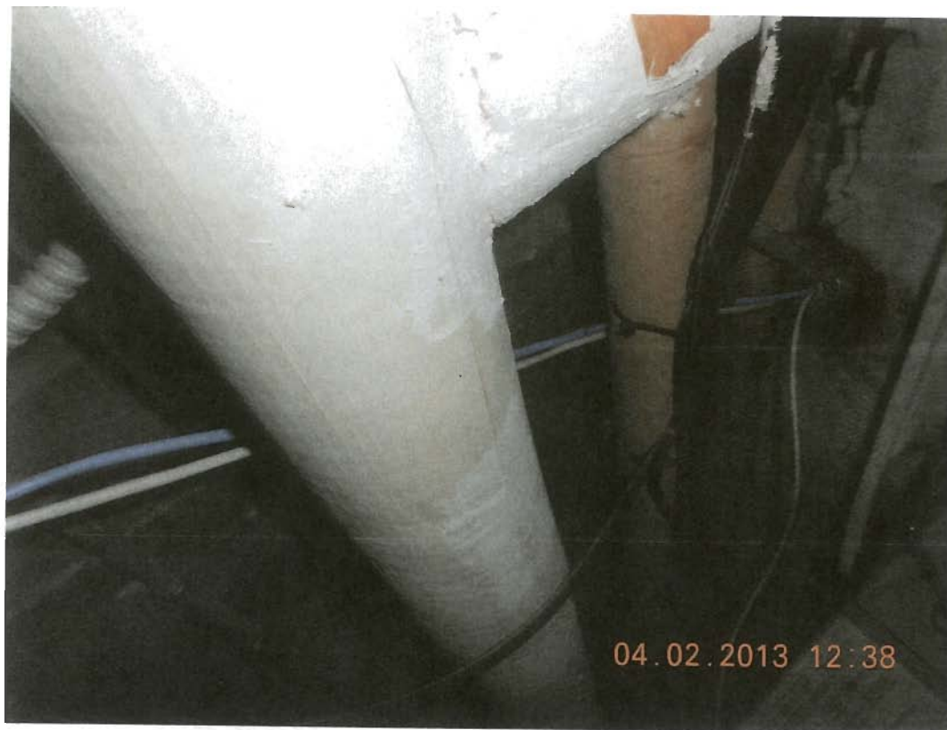
Photo #7 – White mastic on fiberglass
