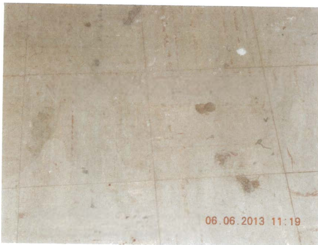
Photo #3 – 9”x 9” floor tile and black mastic – various colors - PACM*
