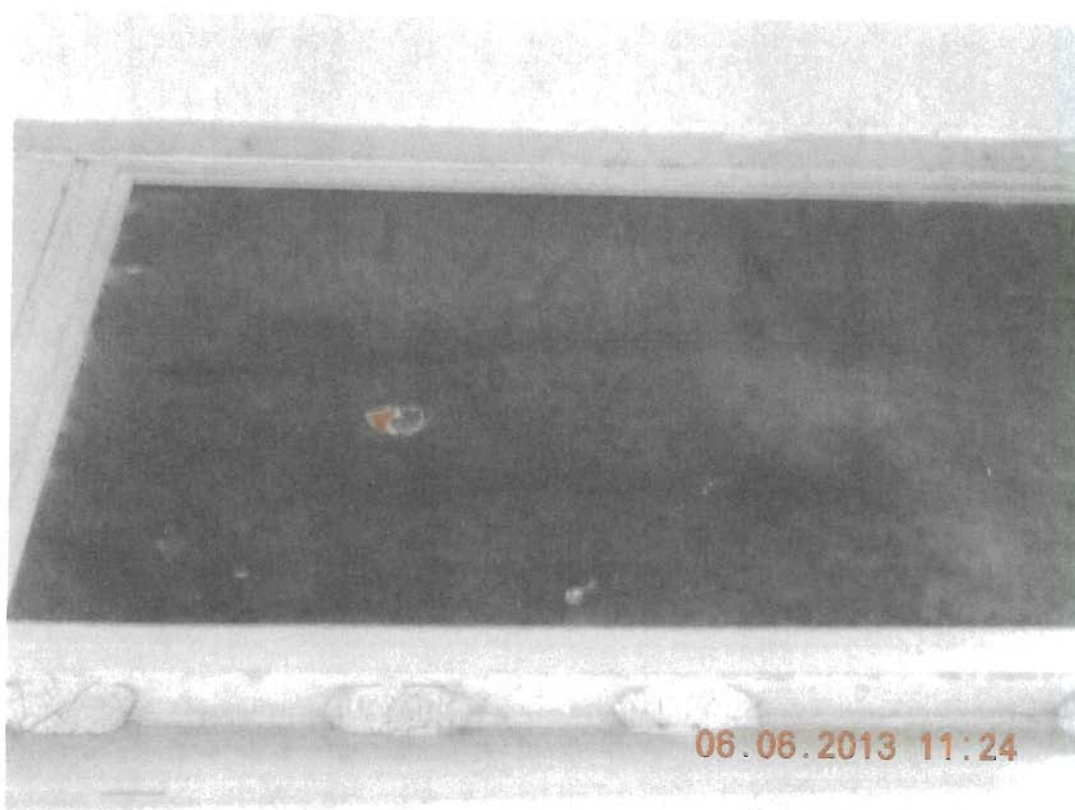
Photo #12 – Transite Panels – exterior under windows – PACM*
