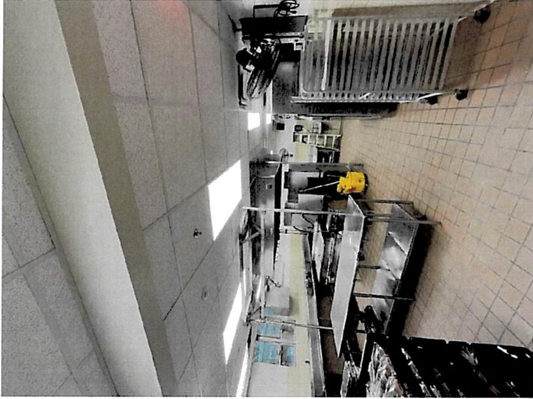
Wrong ceiling tile installed in kitchen, need food service rated tile
