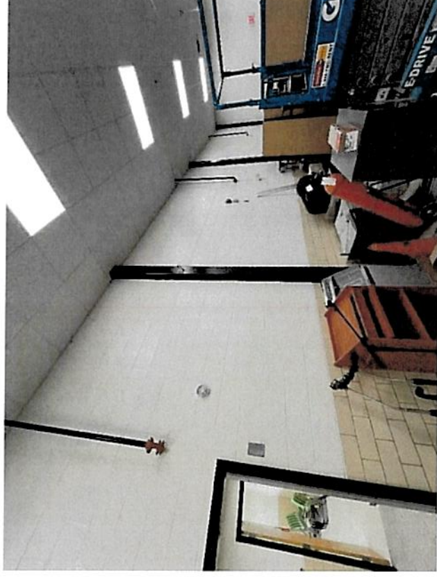
Paint sprinklers lines at stage and back wall of café to match wall
