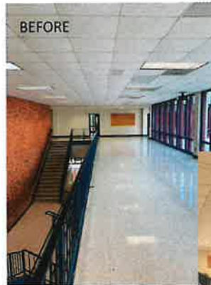
Left: Roof, bulb, and ceiling tiles in need of repair
