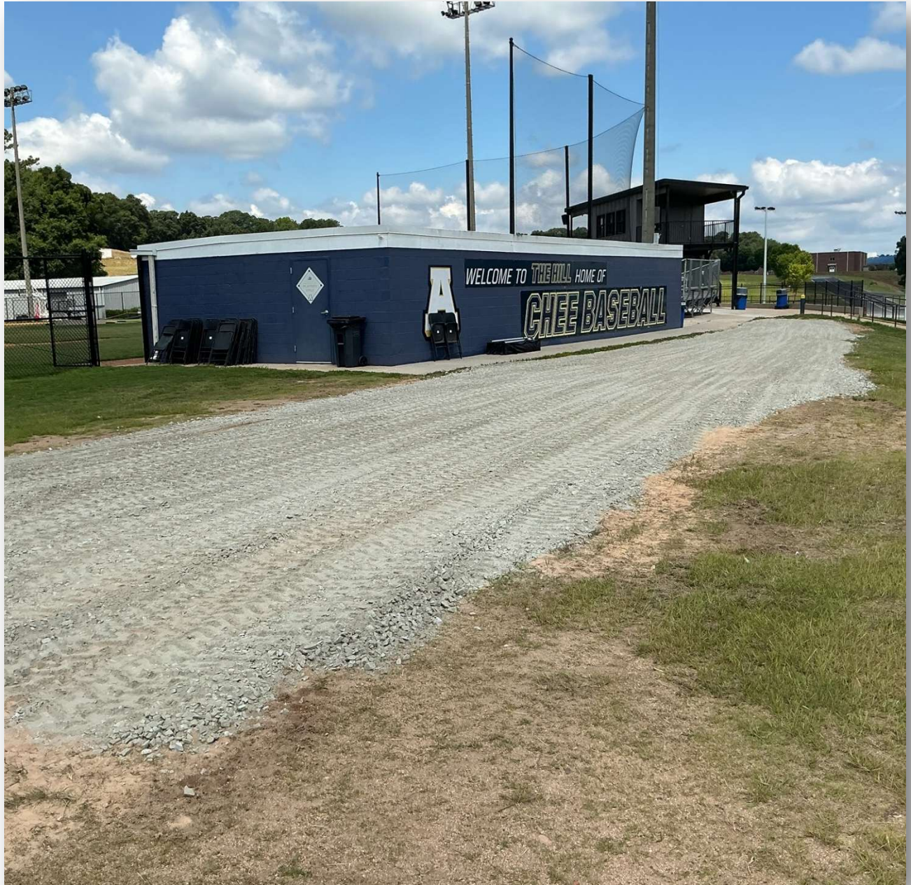
GAB installation at Apalachee baseball drive
