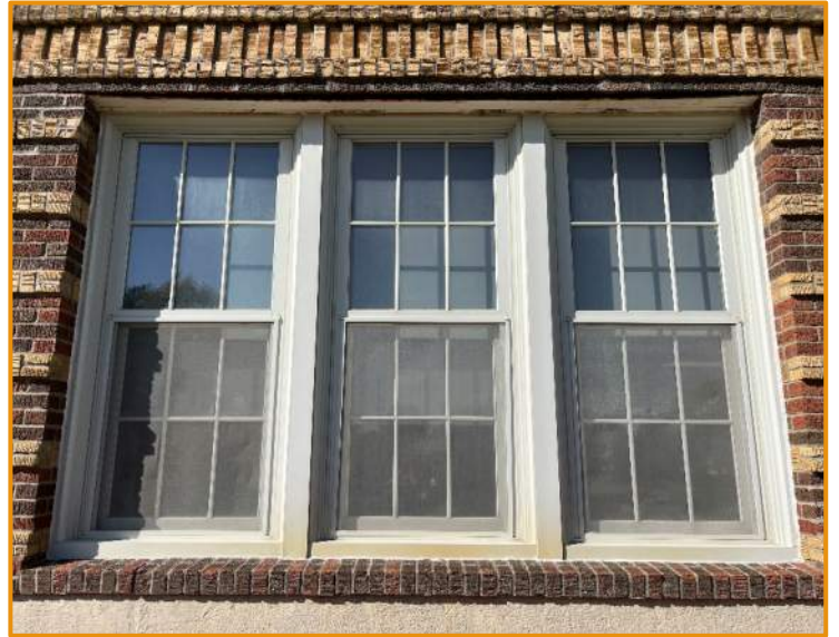
Figure 5: Masonry failure – East sagging brick above window; crumbling brick
