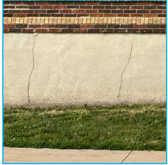
Figure 13: Masonry Failure – See Reference Floor Plan plaster veneer cracking – priority 3
