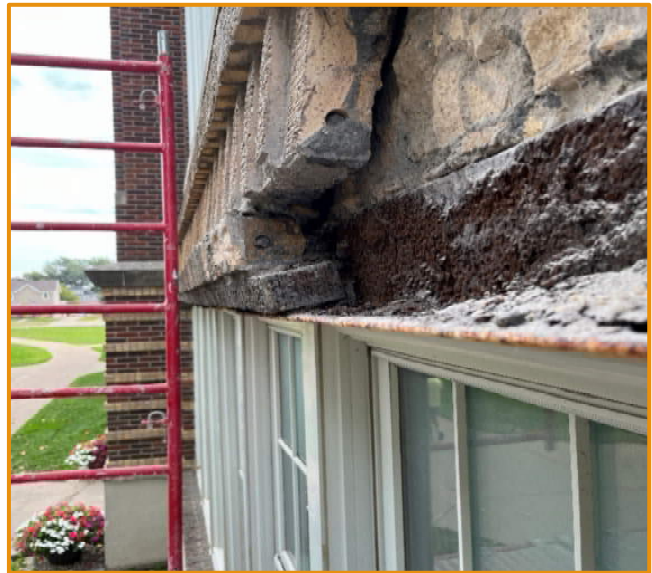
Figure 3: Masonry Failure – Northwest protruding brick; lintel deteriorating
