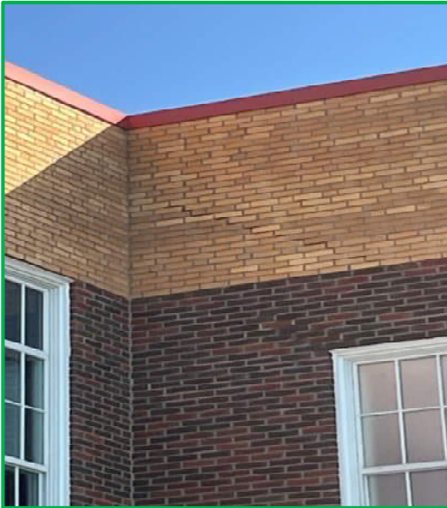
Figure 10: Masonry failure - West stair stepping cracking
