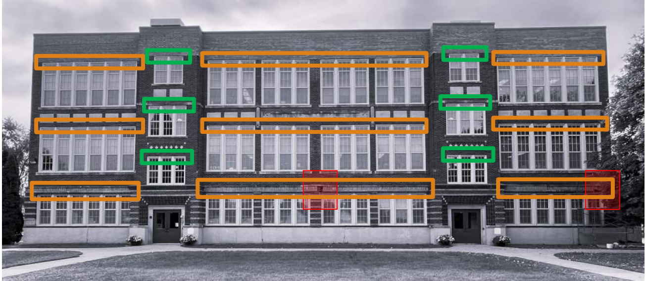
Figure 1: North Façade – Masonry failure locations; Red highlights indicate areas of investigation
