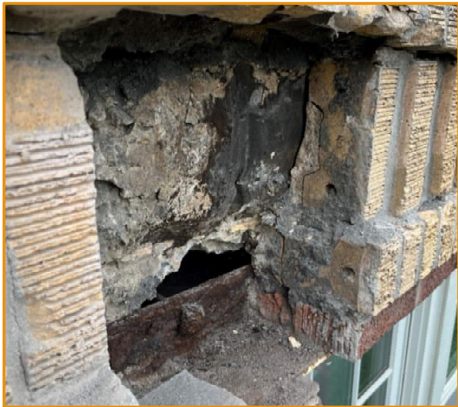
Figure 2: Masonry Failure – North center lintel at library / no concrete beam attachment
