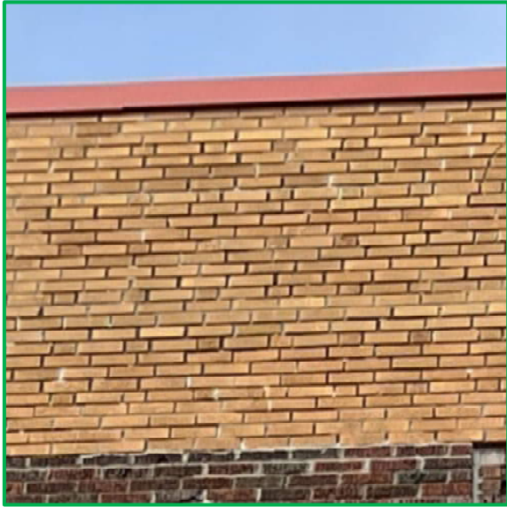
Figure 12: Masonry Failure – Beige Brick Tuckpointing – priority 2
