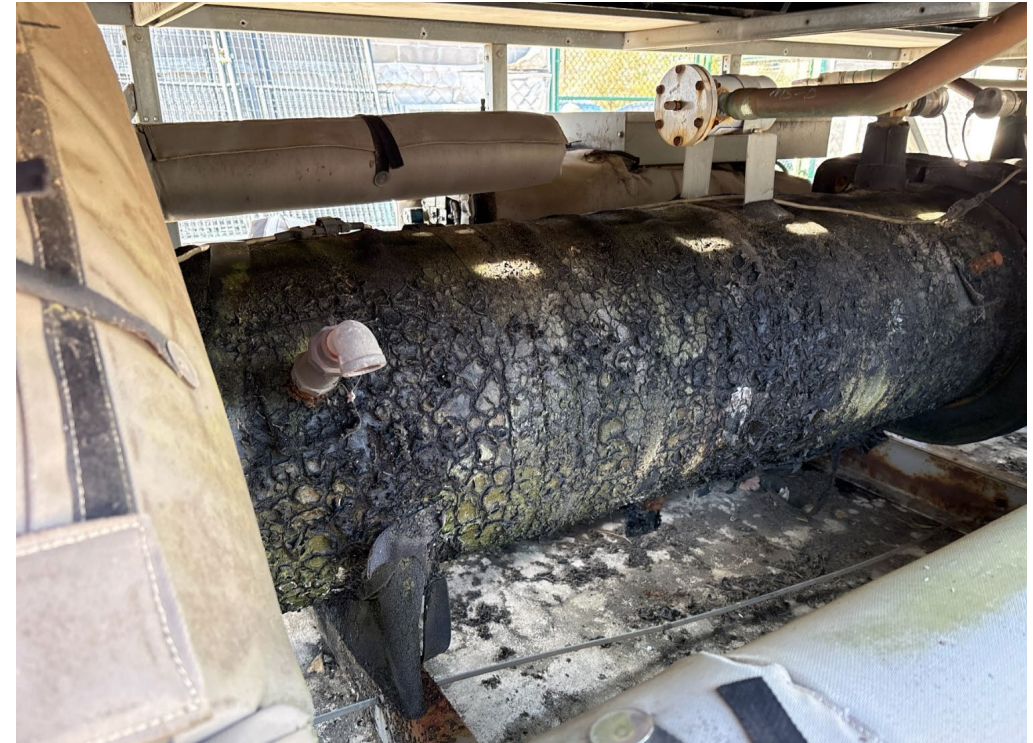
Chiller – Holly Shelter MS
