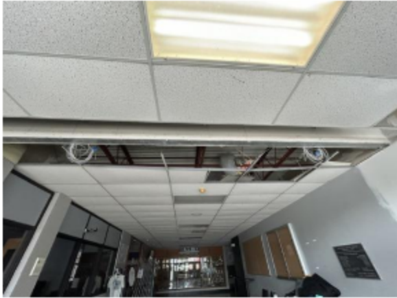
North parking lot control wire
