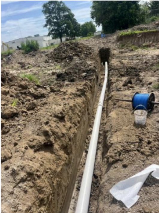
Main Water line
