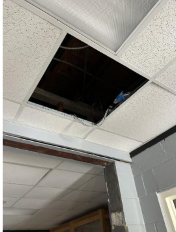
Middle School controls wire
