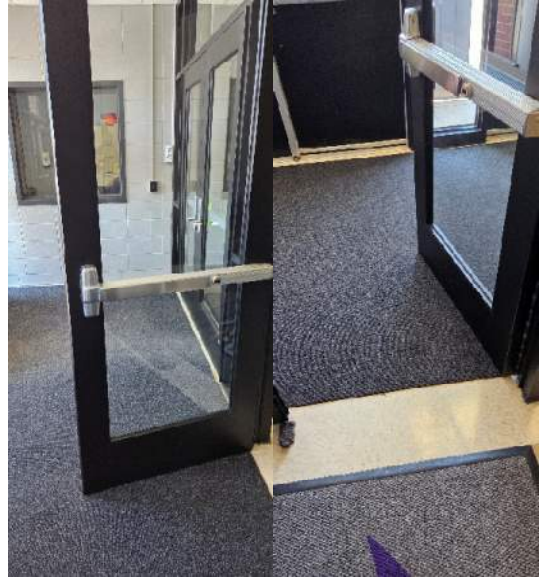
North High School Entrance: Door/Flooring Interference
