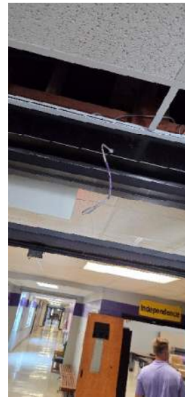
Middle School Entrance: Ceiling Tiles and Camera Wire
