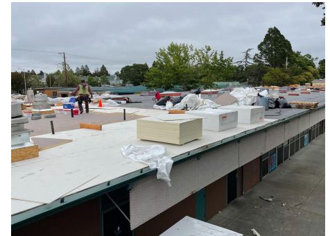
CCLA Roofing & HVAC
