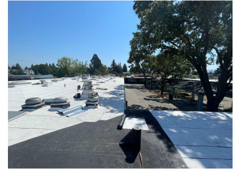
CCLA Roofing & HVAC
